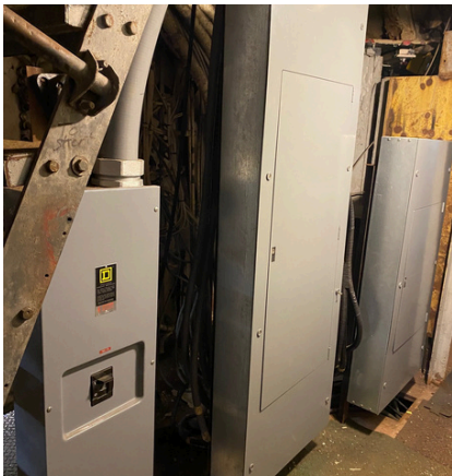
To the left, the breaker panels that were installed when Little Rock came to Buffalo. To the right, the ship's original distribution panel. We're examining if the original panel can be brought safely back into service.
