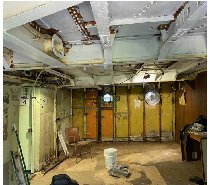
Above: The demo of the Memorial Wardroom continues along with repairs as we find degraded areas along the way. The first coat of metal primer has been applied to the overhead.
